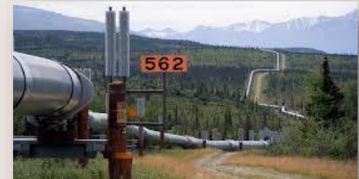
Single pipeline connection
